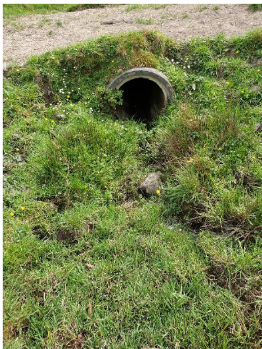
Photo 9. Downstream channel after the culverted farm crossing with pugged ground.
