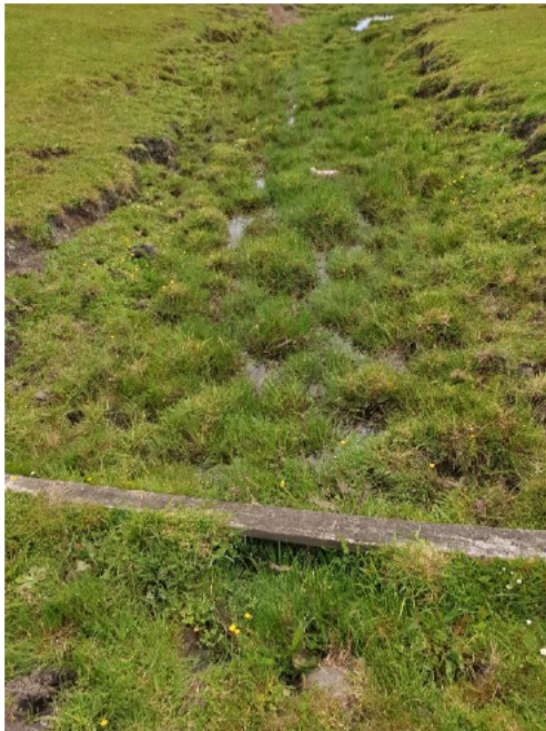
Photo 3. Channel banks are distinguishable however, degraded due to livestock
