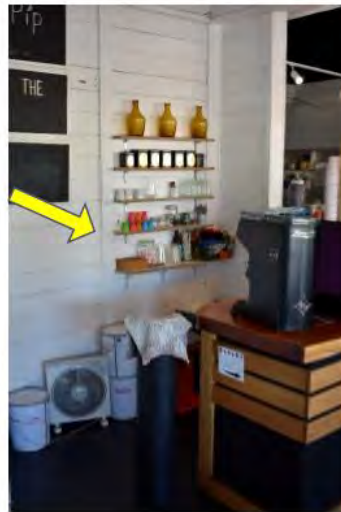
Fig. 15 The vertical batten and slight misalignment of the interior panels suggests that there may have been previously an opening within the back wall of the store.
