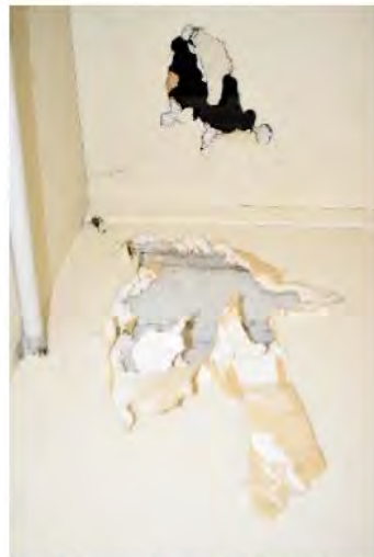
Fig. 17 An area of damaged GIB plasterboard from the space behind the front of house revealed an exterior weatherboard cladding suggesting the extent of the original building and store.
