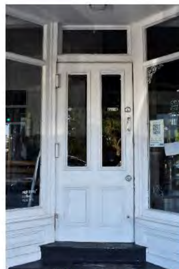
Fig. 31 The existing door and transom window of the café display similar architectural details that can be seen in the c1890s photograph suggesting these to be original features.
