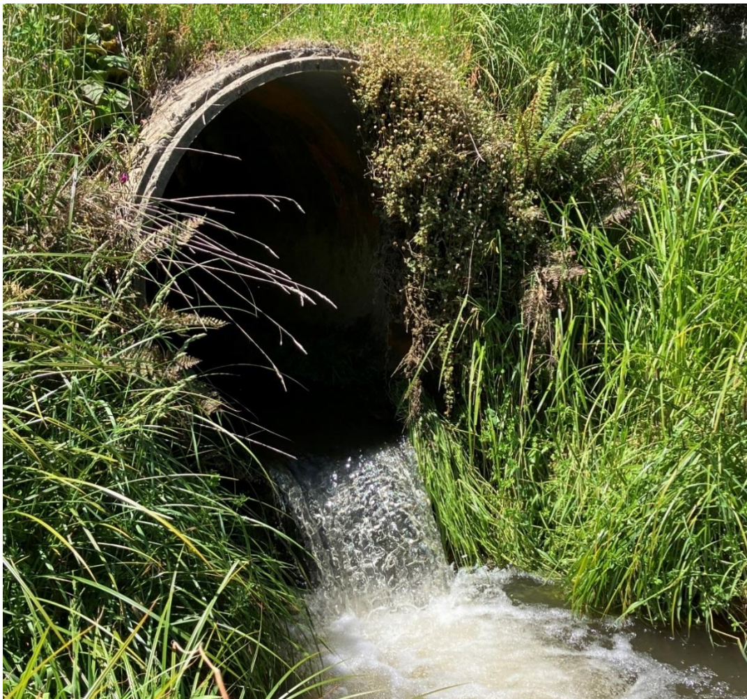
Plate 1: Downstream end of the perched culvert identified at Site 2.
