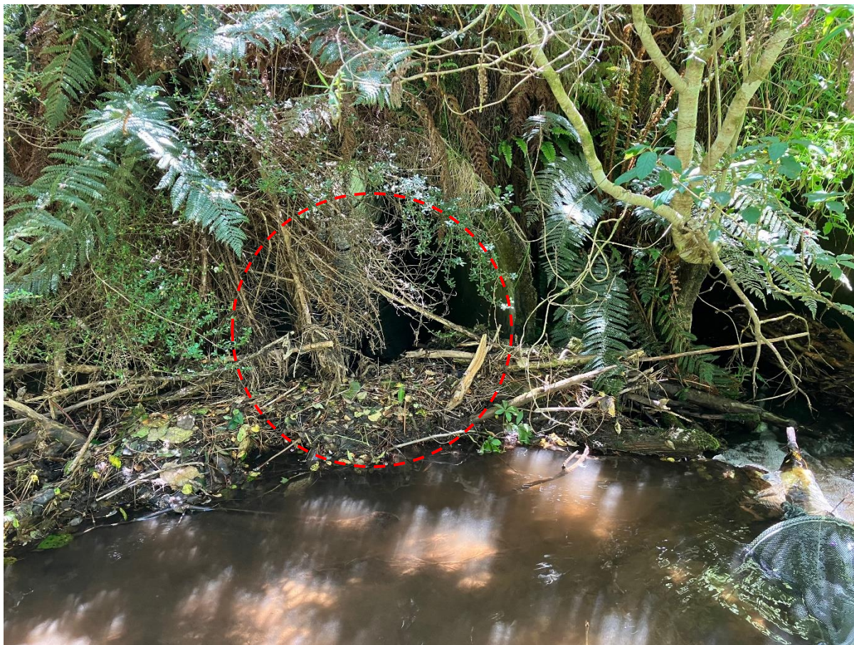
Plate A2.5: Debris build-up at the upstream end of the triple barrelled culvert at Site 4, this will restrict fish passage and has caused a small fall to develop, directing majority of the stream flow down the right most barrel. Dashed outline indicates the approximate location of the central culvert barrel.
