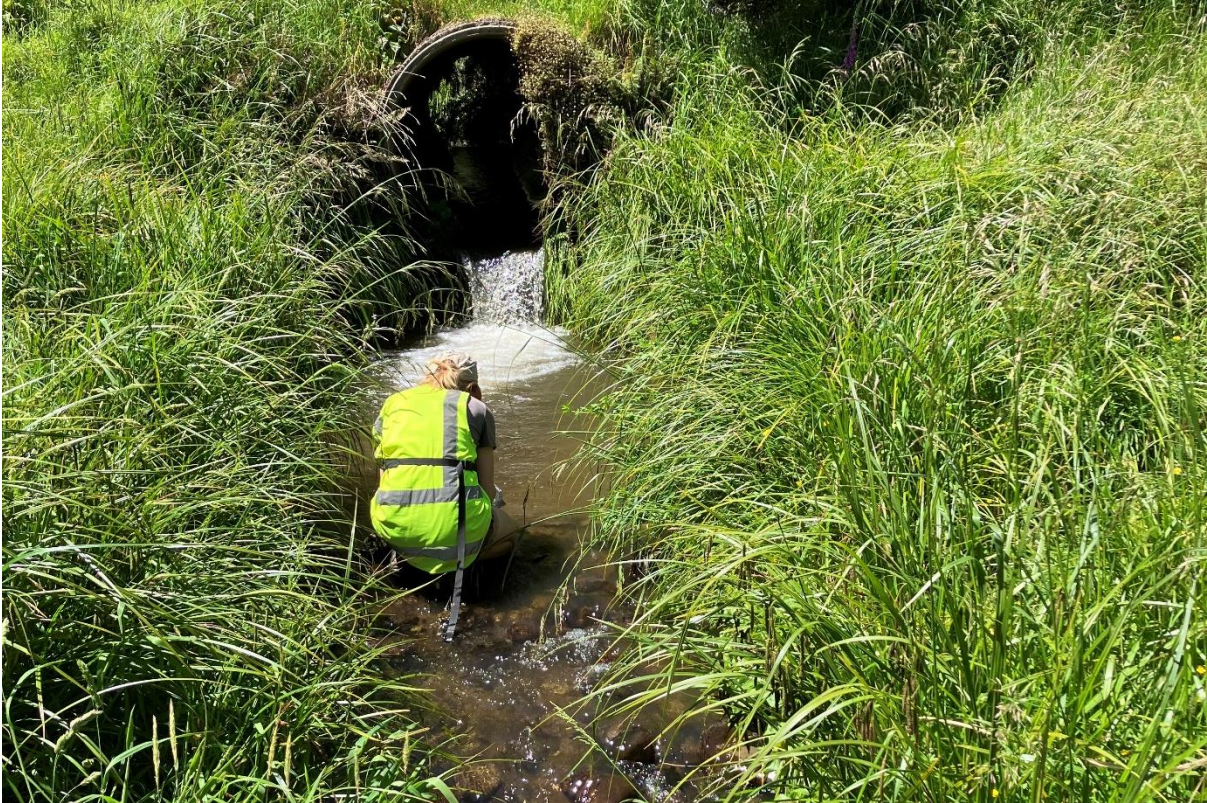
Plate A2.3: Site 2 perched culvert.
