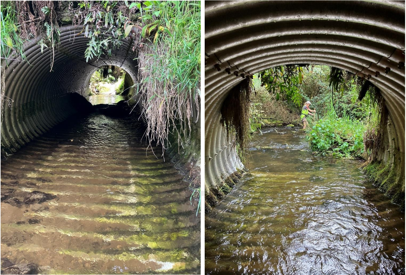
Plate A2.4: The culvert at Site 3 is an example of a fish-friendly structure. Views looking upstream (left) and downstream (right) from within the culvert. Width of the culvert is approximately that of the stream, and is in line with the stream both in and out. The water is a similar depth and velocity within the culvert as it is in the stream, and a small amount of bed material has collected within the culvert.
