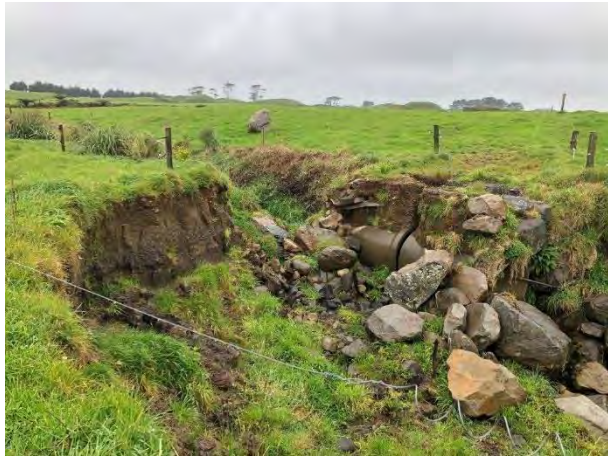
Photo K: Erosion around a culvert crossing within stream S5.
