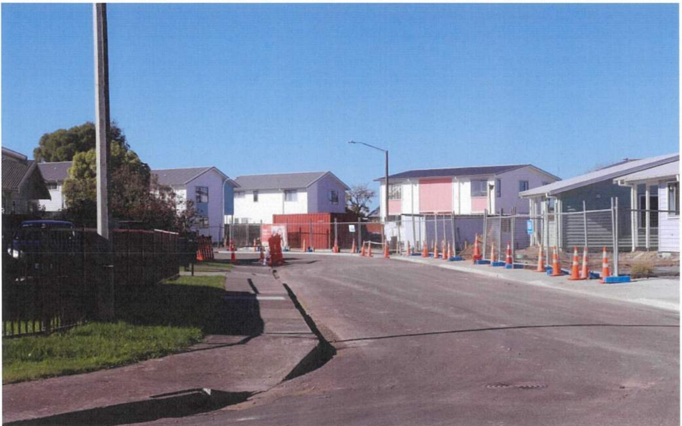
Kāinga Ora homes under construction in Mahora, Hastings. Photo: RNZ / Tom Kitchin
