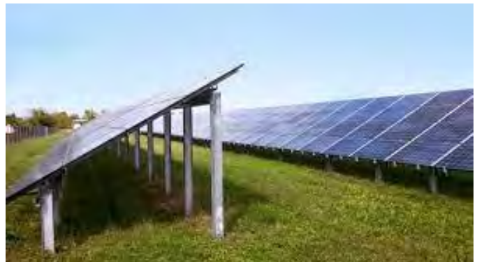
Fixed tilt solar farm
