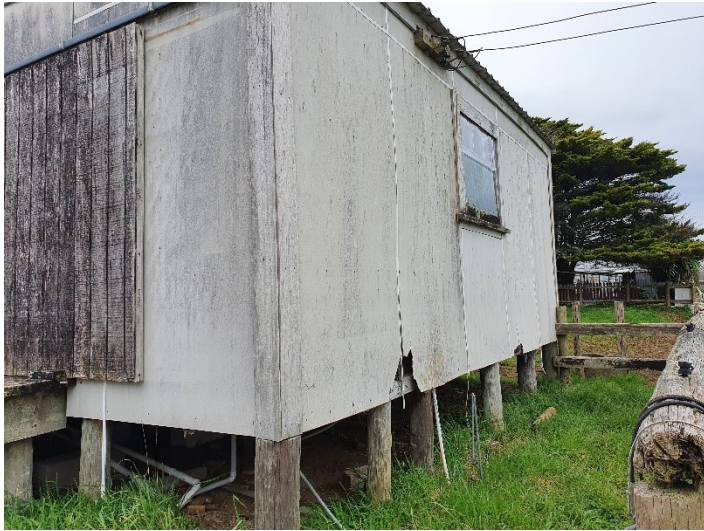
Stables (2) - Minor Damage to PACM Cladding
