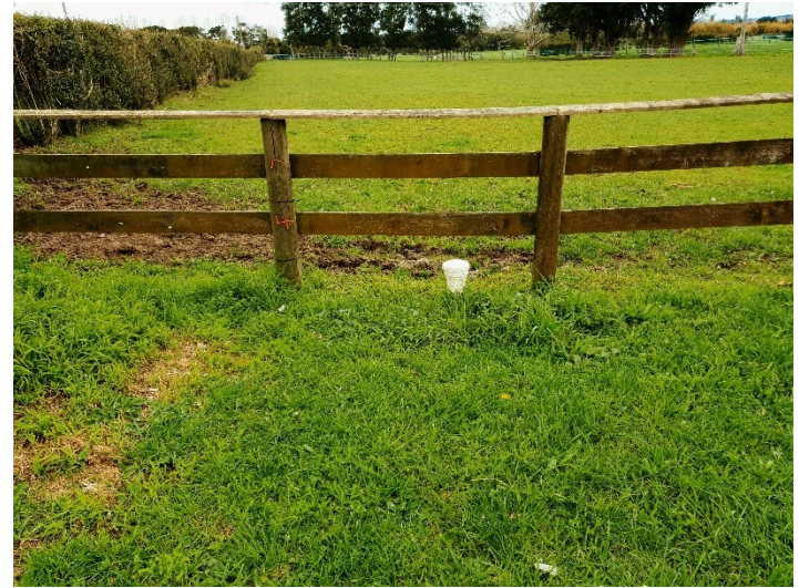
Septic Tank Vent
