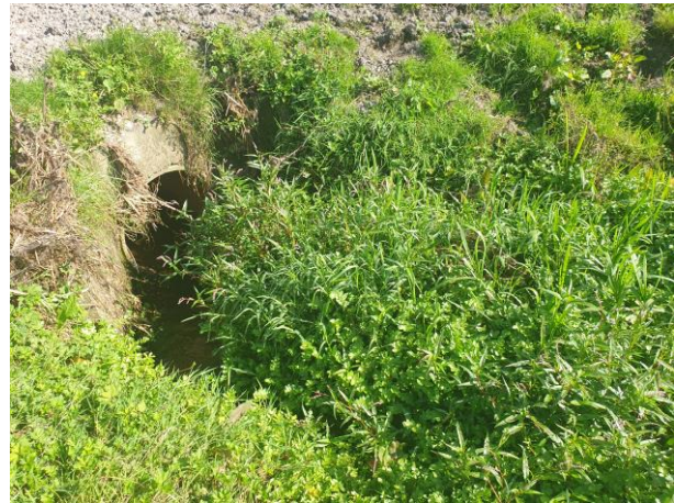
Photo 47. The natural inland wetland discharged to Watercourse 2 through an undersized culvert.
