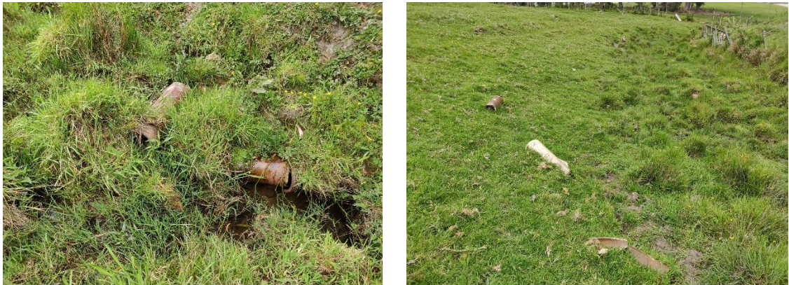
Figure 17. Sections of unmarked glazed ceramic drainage found along eastern creek of 98-100 Totara Road
