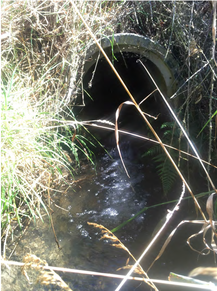
Figure 8. Perched culvert in the roadside waterway and tributary of North Brook.
