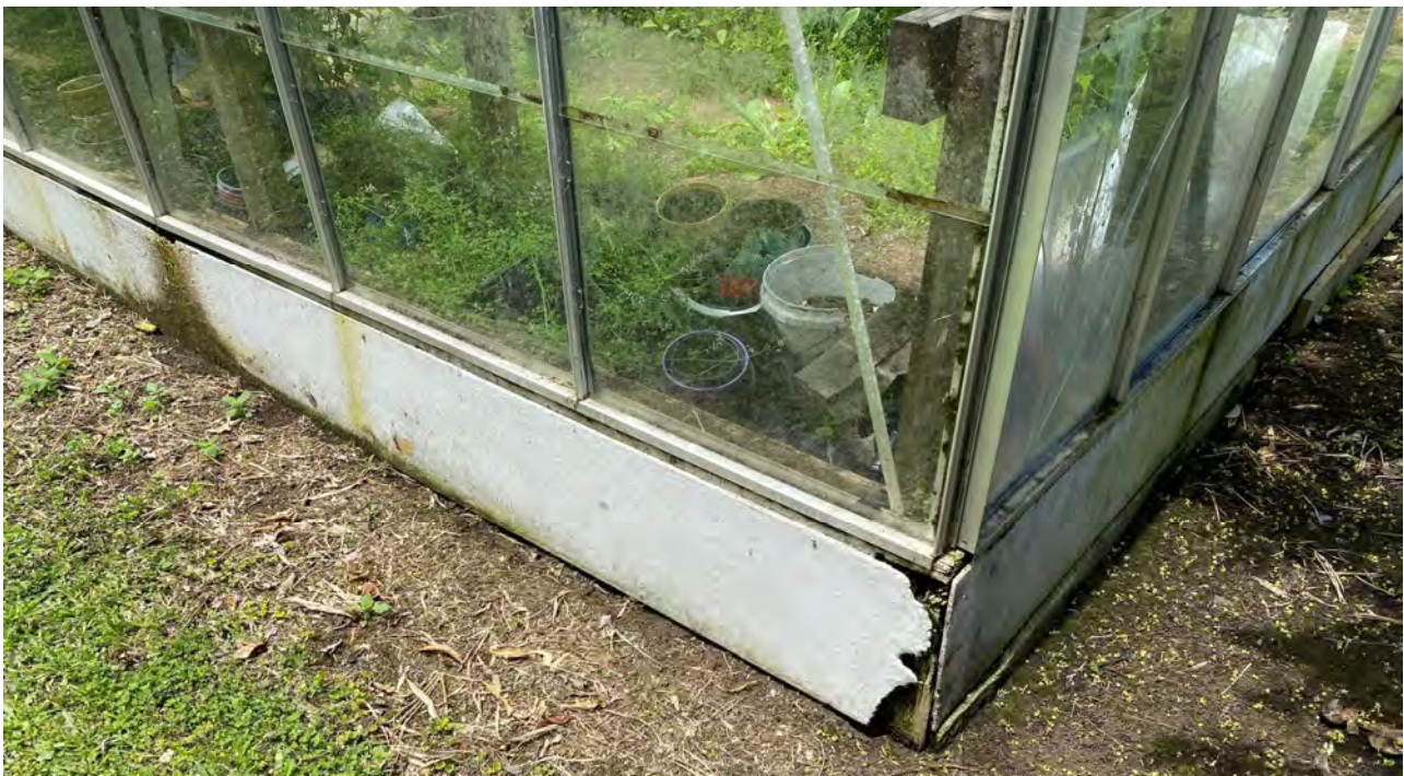
Figure 7. Deteriorated cladding of glasshouse.
