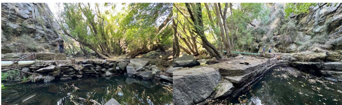
G. The downstream (left) and upstream (right) side of the Lower Gorge weir. With no finer gravels/sediment to seal the structure, water is flowing through it.
