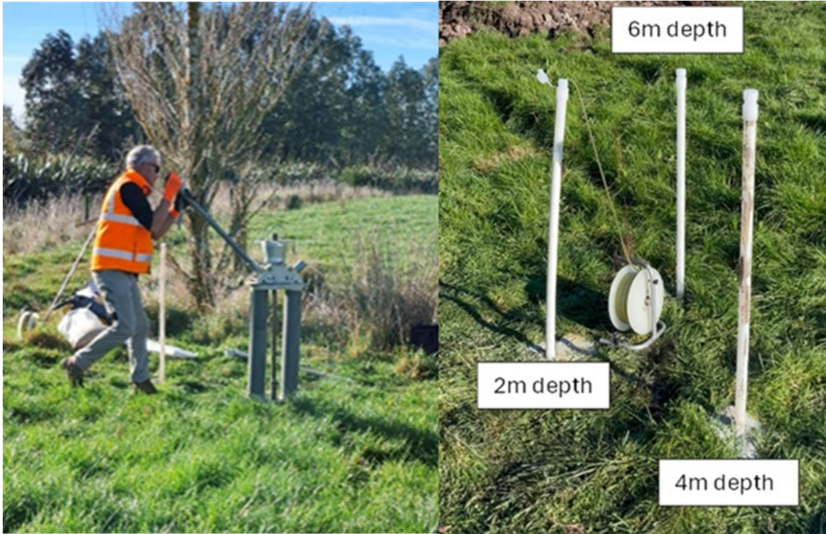
Figure 9 Extraction of steel casing (left), and piezometers installed at various depths on the Pamu Landsdown farm during the field day.
