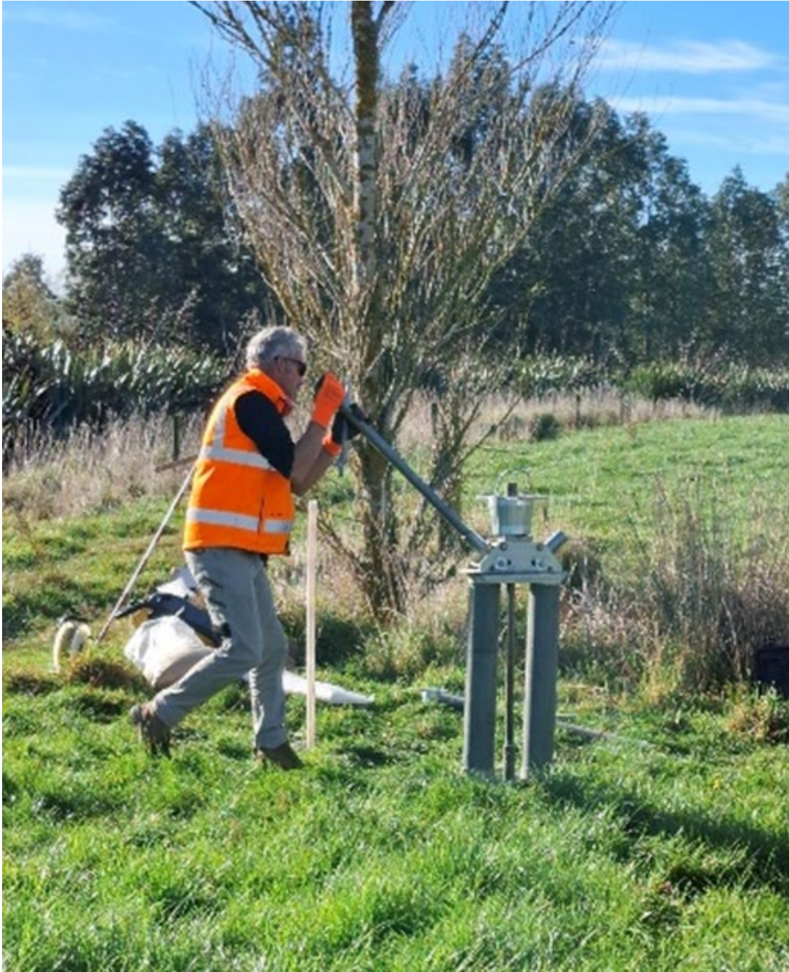
Dirk Van Walt (Van Walt NZ), installing a direct push piezometer at Landsdown during the field day
