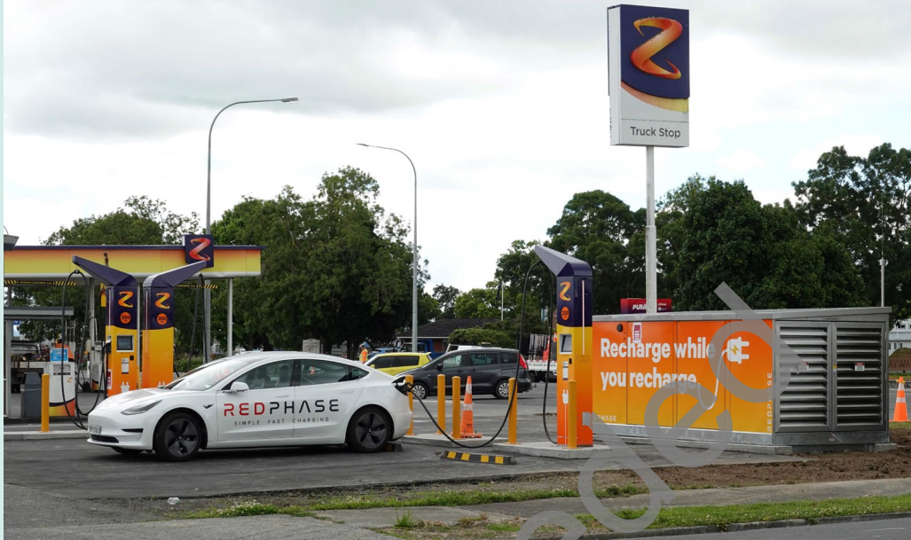
Image: The Kwetta charging point at Z Energy in Ngātea
