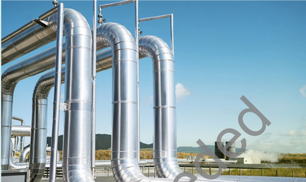
Image: Pipes at Ngā Tamariki geothermal station
