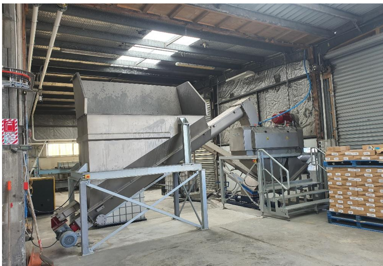
Photo: Installed depacker at Prime Environmental Christchurch facility. Source: Prime Environmental
