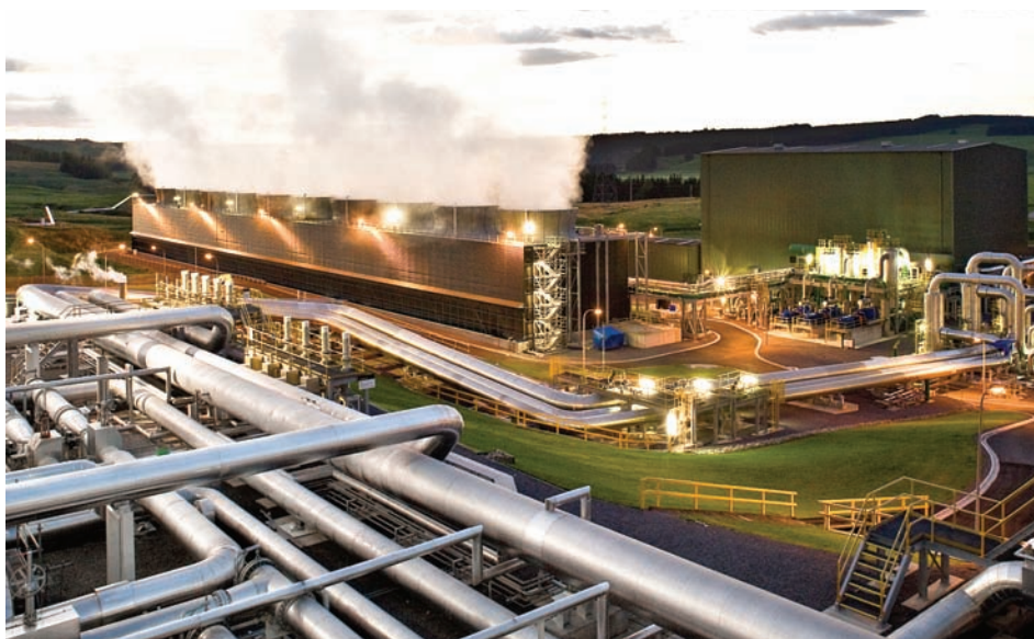
(Photo courtesy of Mighty River Power)
