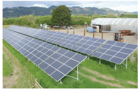
Figure 16 Ground-mounted PV array, Drury, Auckland
