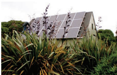
Figure 23 Roof-mounted PV array
