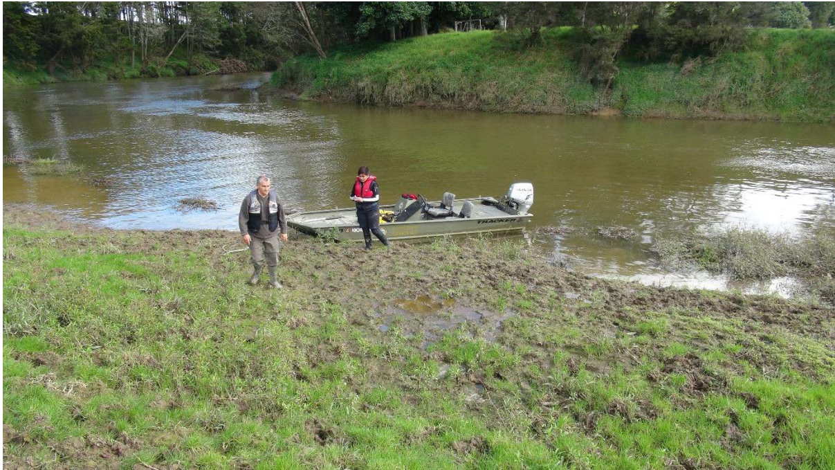
Figure 1 Example of stock damage to a river bank in the Kaipara catchment, Northland, August 2016 (photo: Millan Ruka)
