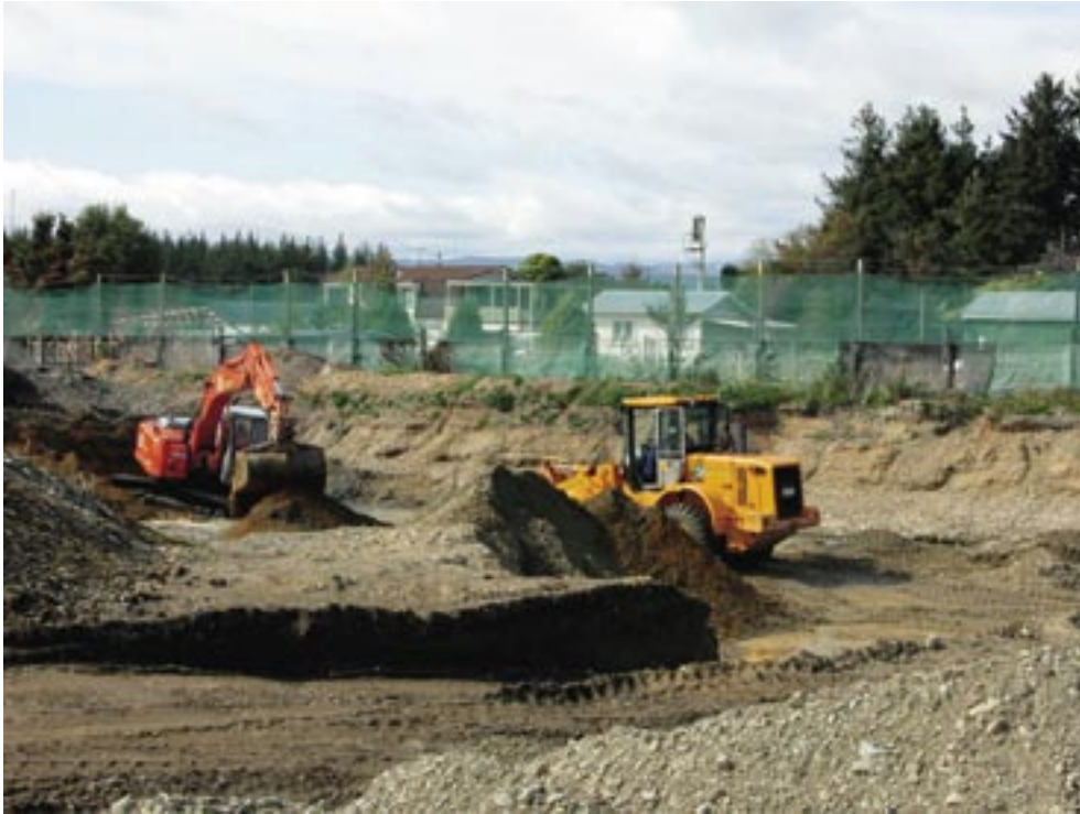
The clean-up of New Zealand's most contaminated site – at Mapua near Nelson.
