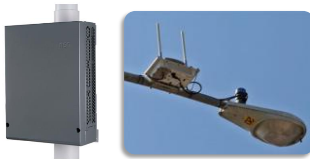
Figure 5: Example of a small-cell unit (left) and a pico-cell installed on top of a lamp-post (right)
