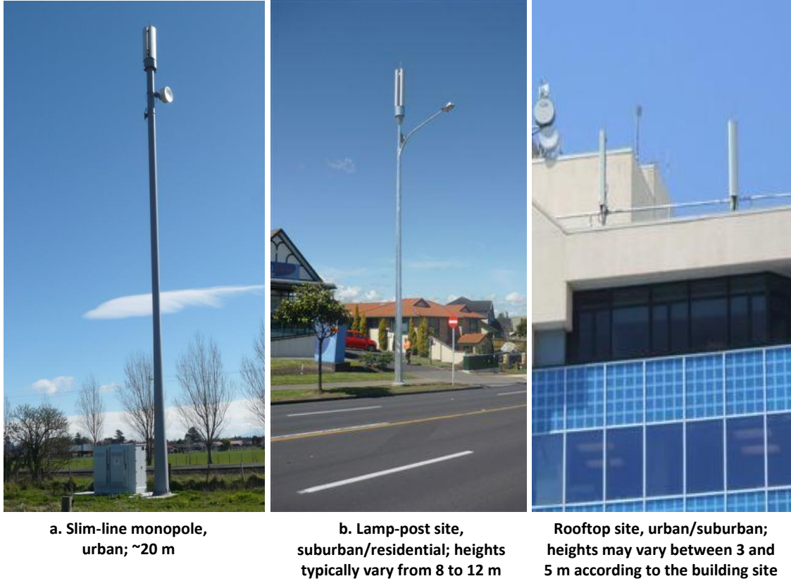
Figure A2.10: Examples of different installed antennas
