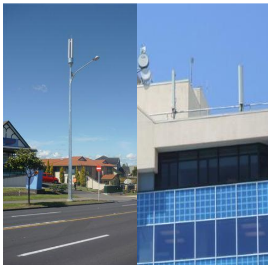
Figure 2: Examples of different mobile network antennas (in the photo on the right, the two structures are telecommunications antennas)
