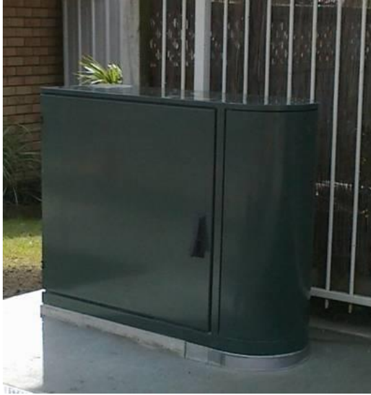
Figure A2.14: A fixed network street cabinet
