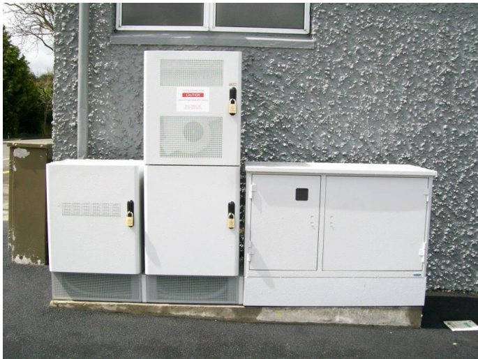
Figure A2.13: Cabinets installed by 2degrees NZ Ltd
