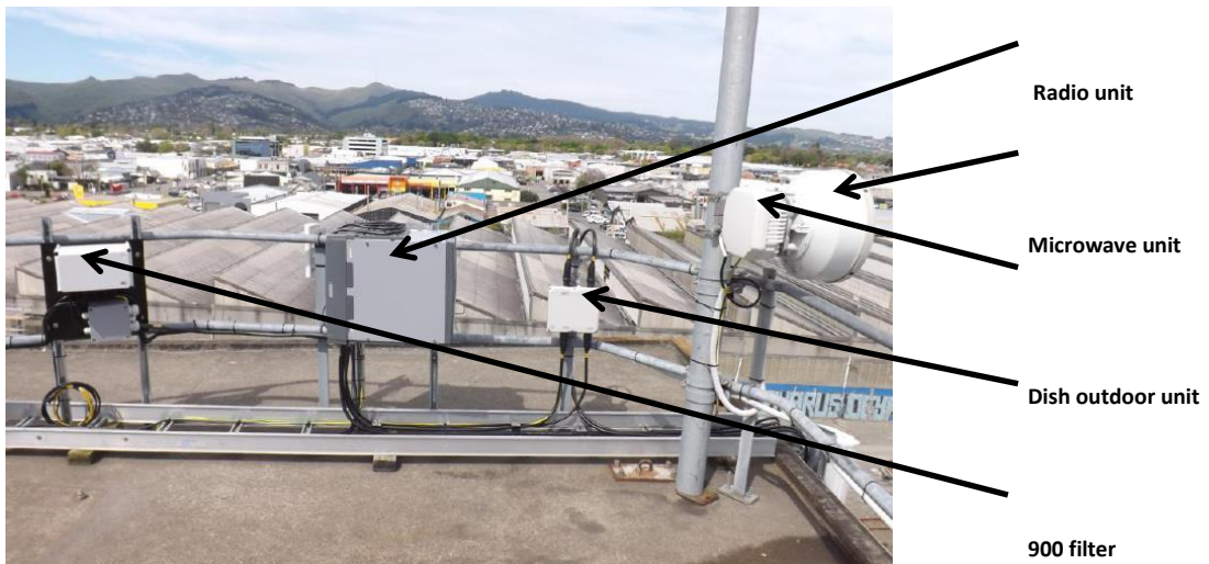
Figure A2.15: Examples of ancillary equipment installed on a roof-top site
