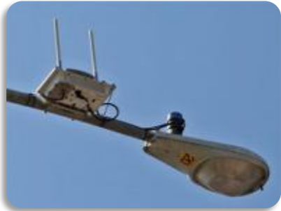
Figure A2.12: A pico-cell installed on top of a lamp-post
