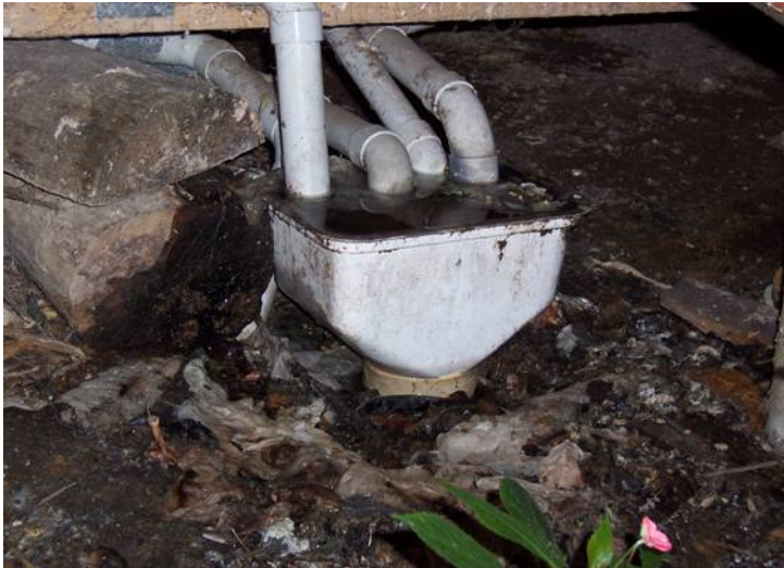
Figure 4: An overflowing gully trap due to inadequate maintenance
