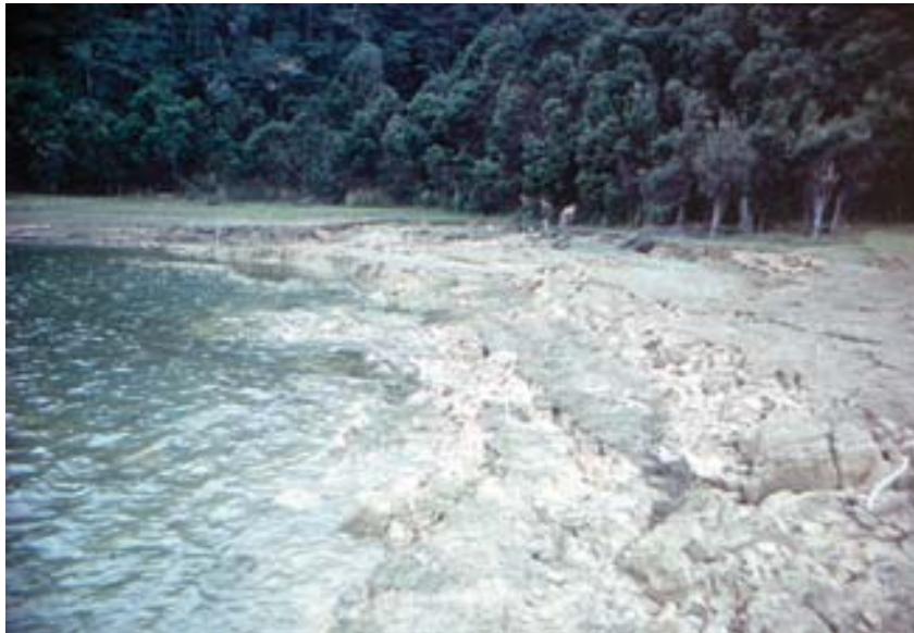
Figure 9: Localised but serious rotational slumping of the lakeshore at Surprise Bay, Lake Manapouri, Fiordland, apparently caused by the lake being drawn down at a faster than natural rate to a level 80 cm below its natural minimum level for a short period in August 1972. (3 March 1973; lake level 176.39 m.)
