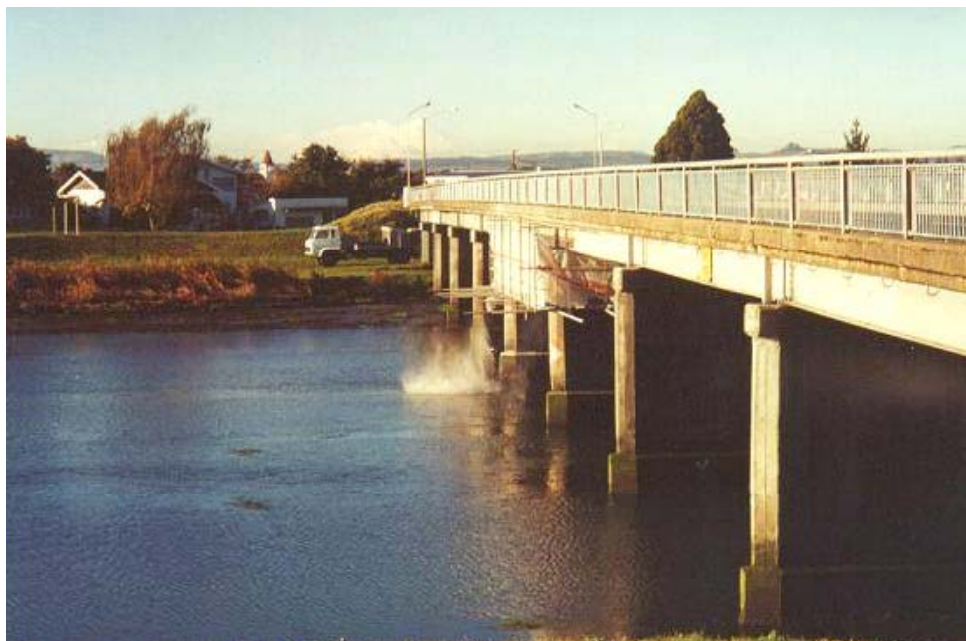
Figure 4.1: Illustration of dust impacts of sandblasting a bridge in the Hawkes Bay region
