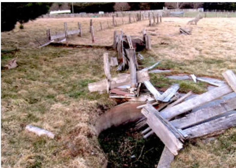
Figure A.10: Former pot dip with large, partially collapsed, holding yards
