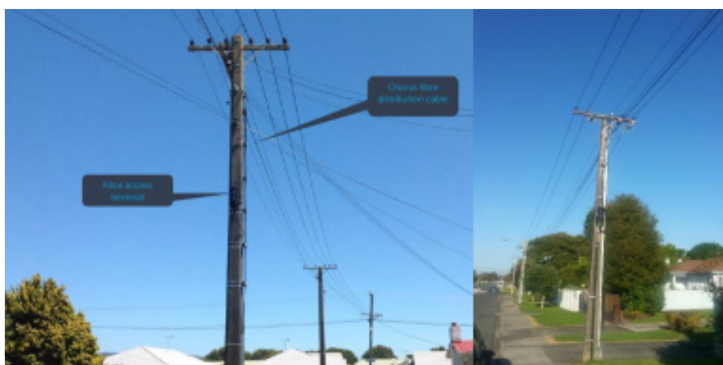
Figure 11: Aerial telecommunication lines
