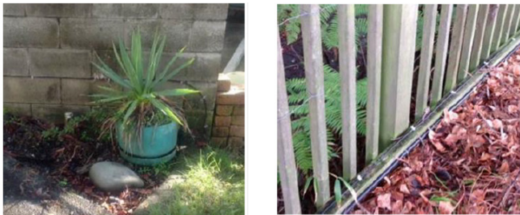
Figure 10: Surface-mounted customer connection lines
