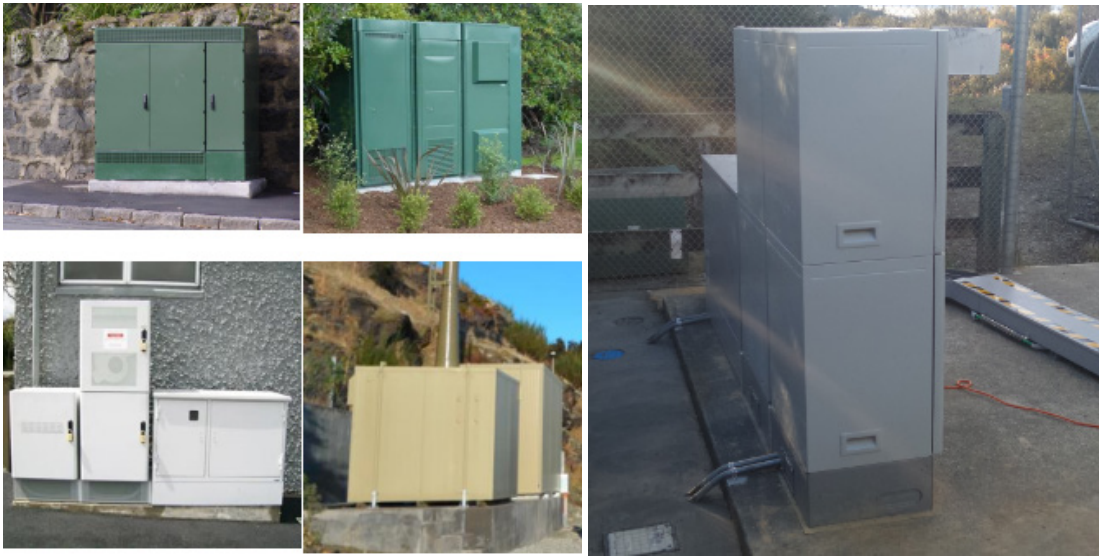
Figure 7: Examples of cabinets in and outside the road reserve
