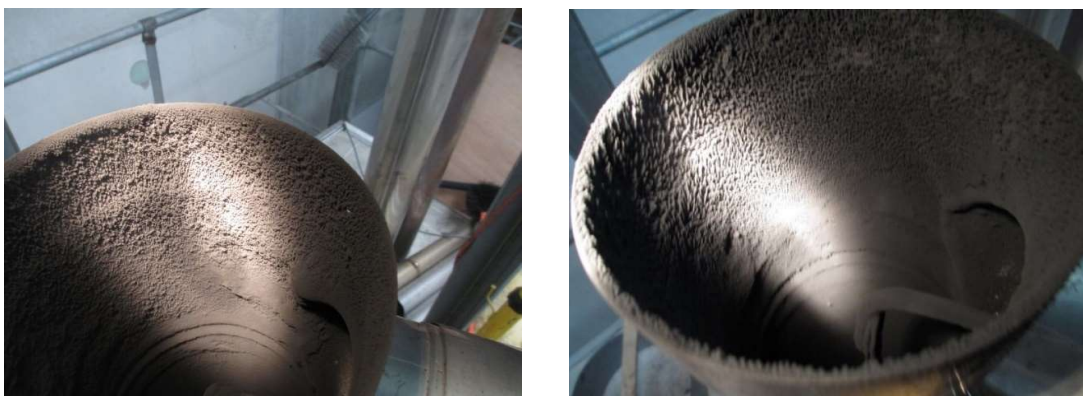
Figure 1: Inside of OekoTube After Operation
