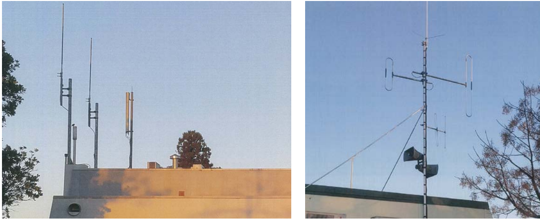
Figure 12: Examples of other non-dish antennas
