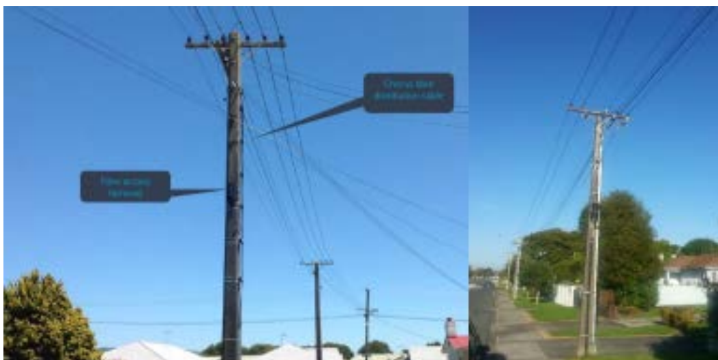
Figure 10: Aerial telecommunication lines
