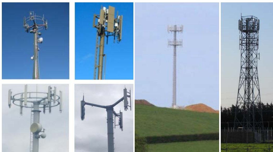
Figure 3: Examples of headframes attached to a pole
