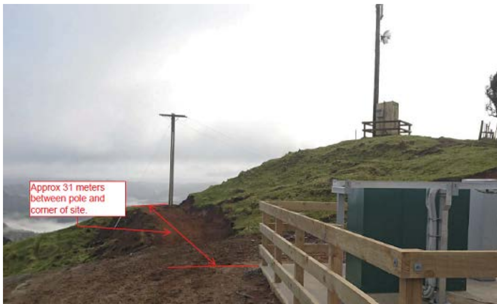
Figure 14: Power supply to telecommunication cabinets in rural site
