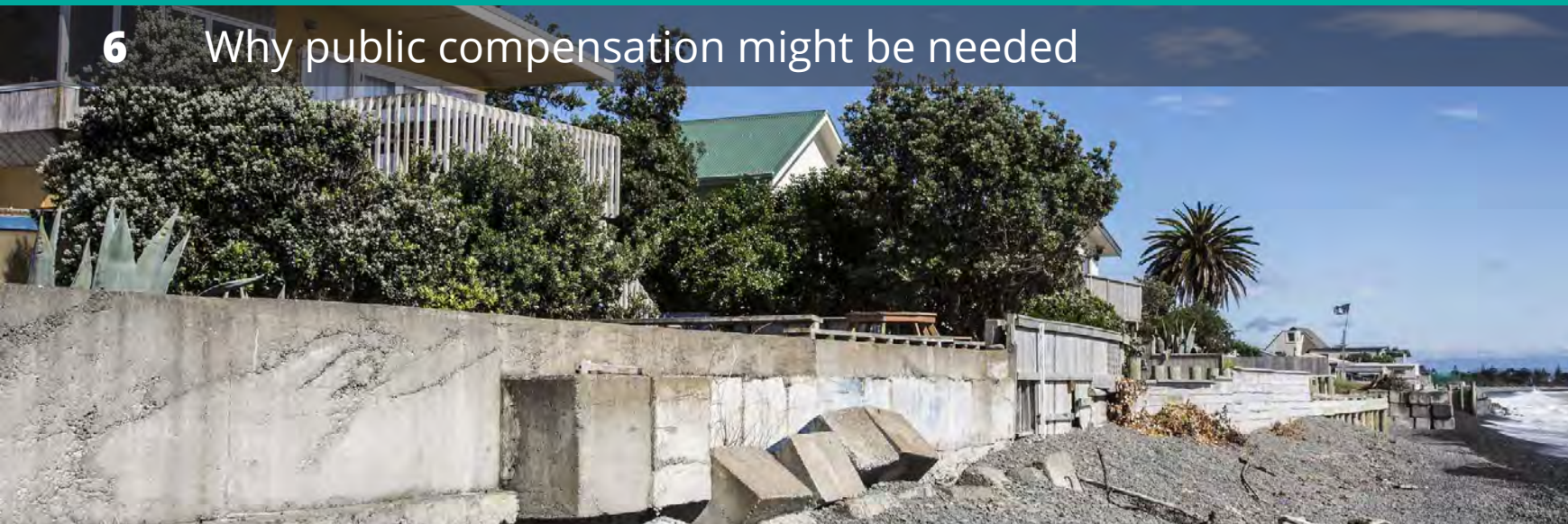
Severe coastal erosion at Haumoana
