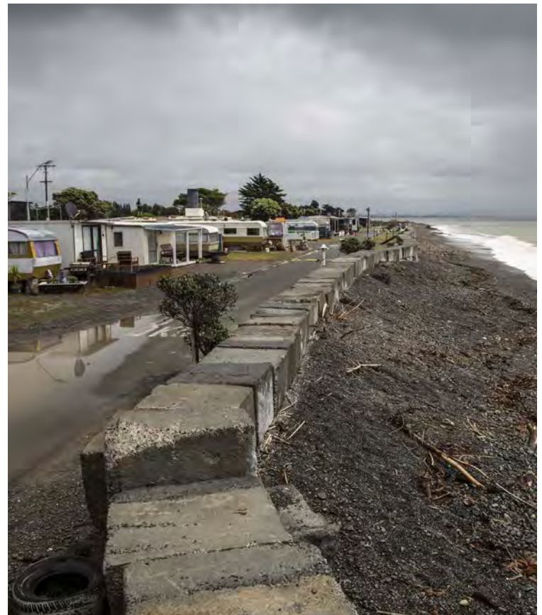
Coastal erosion impacting the Clifton Motor Camp
