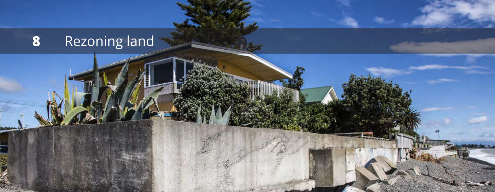
Coastal erosion at Haumoana
