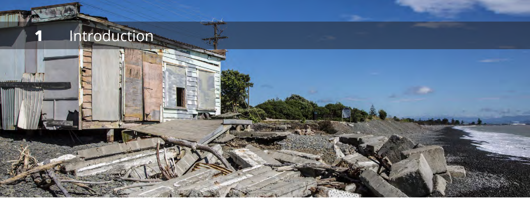
Coastal erosion damaging a house at Haumoana
