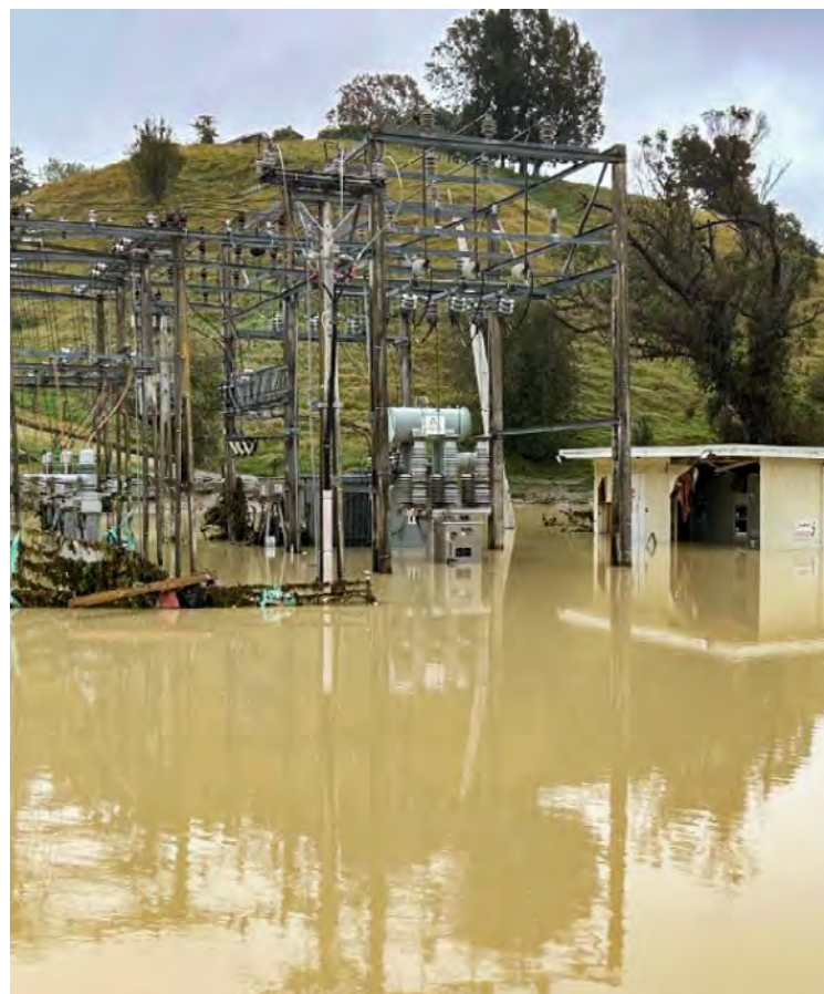
Flooding of Esk Valley substation (Waka Kotahi)
