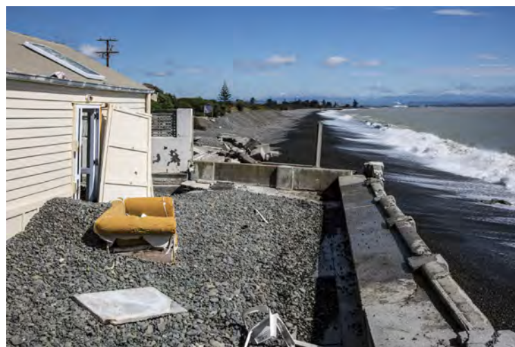
Coastal erosion damage at Haumoana
