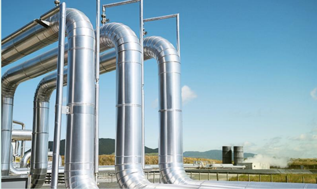
Image: Pipes at Ngā Tamariki geothermal station
